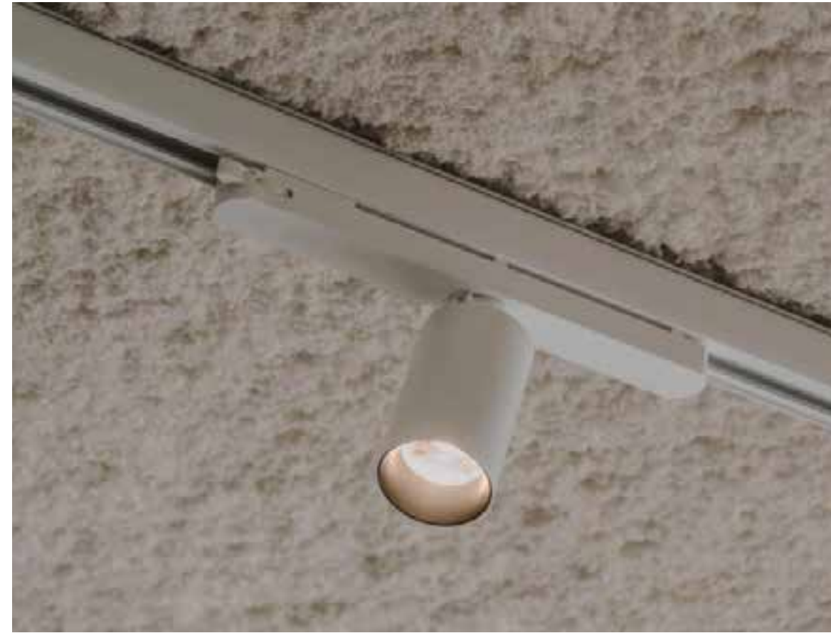
Indoor technical lighting
